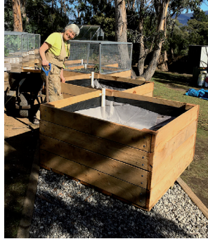
New boxes built and installed in 2020 shown lined with weed mat as a first protective layer and being fitted with wicking bed components: water inlet pipe, pond liner and Geotextile before adding soil and planting out.
